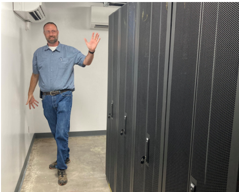
Shak Powers in the new fiber carrier neutral location (CNL) funded by DOLA and matched by La Plata County
